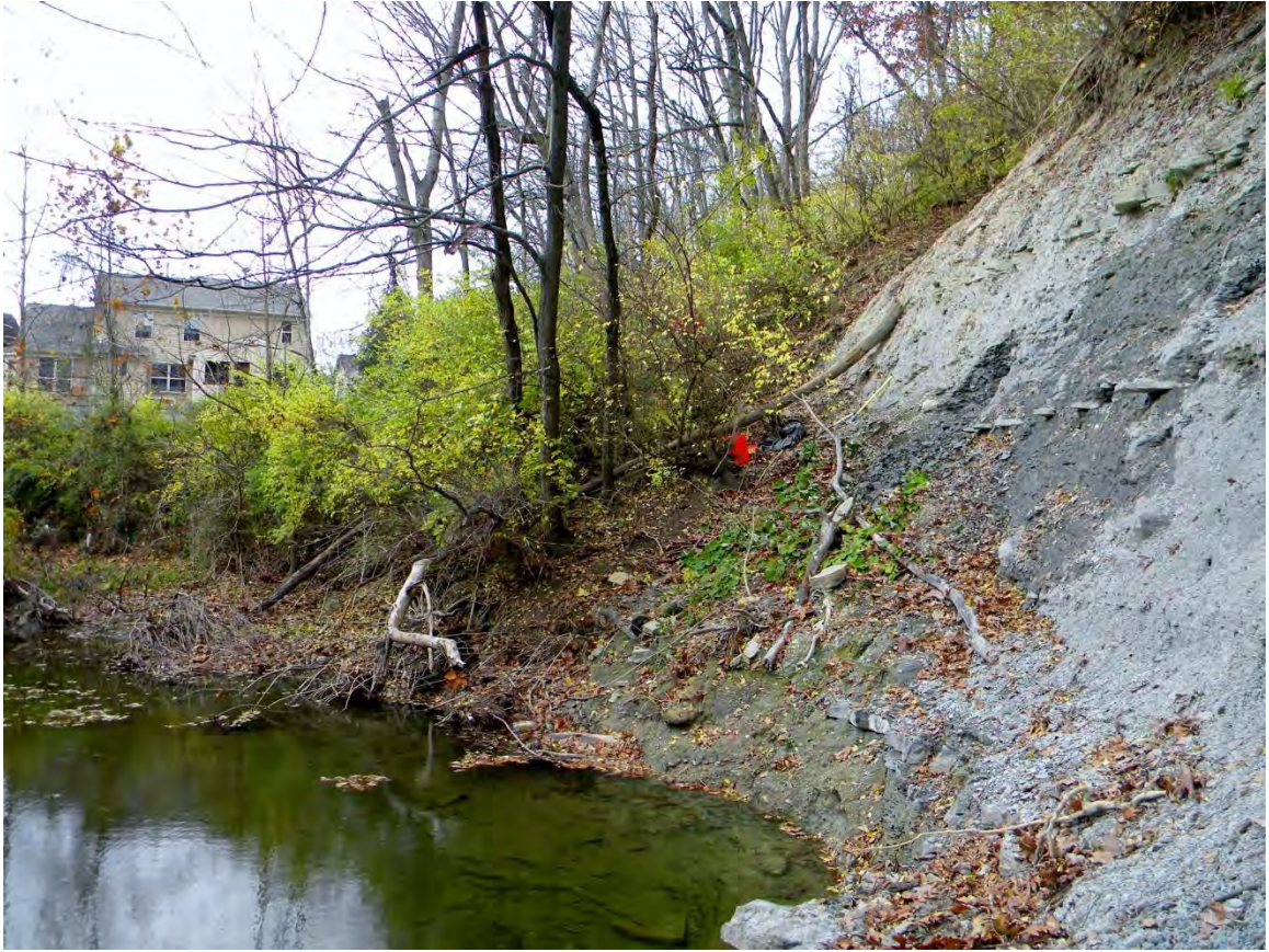
Figure AV.26: Scarp and toe of the Berkshire Road landslide. Notice the accumulation of landslide debris in the toe area.
