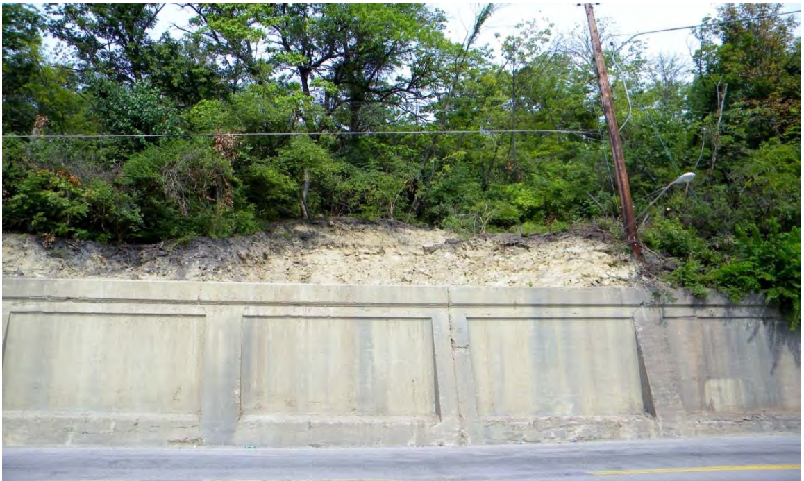
Figure AV.29: Toe of the Columbia Parkway landslide, emerging on the top of the retaining wall.
