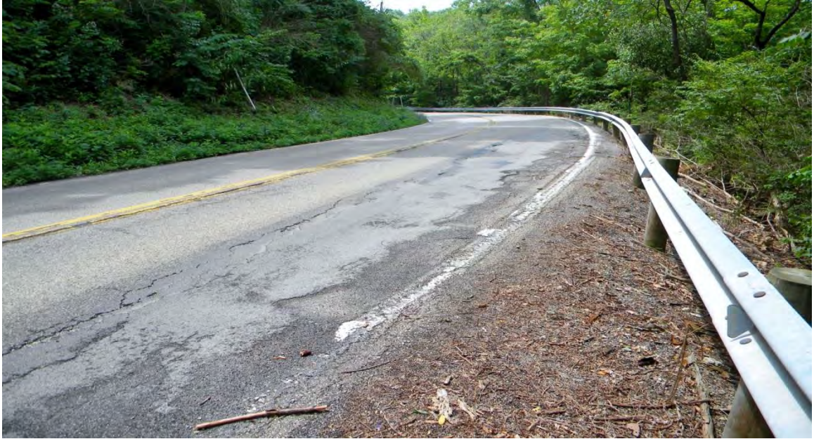
Figure AV.14: Damage caused to Nordyke Road by landslide activity.
