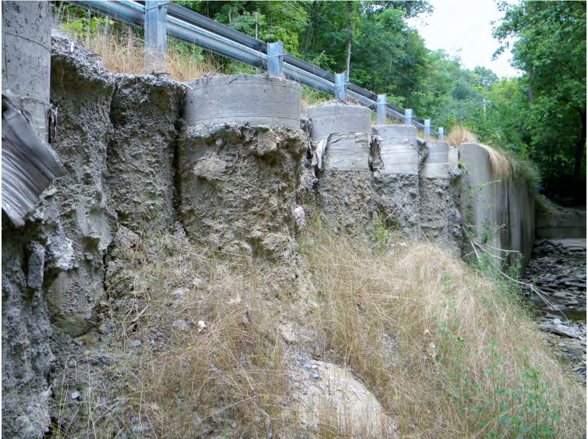
Figure AV.22: Remains of a retaining wall that had been constructed to stabilize Wagner Road.
