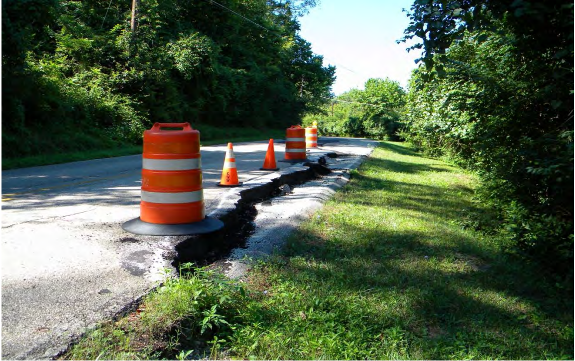
Figure AV.11: An example of the damage caused to Elstun Road as a result of landsliding.
