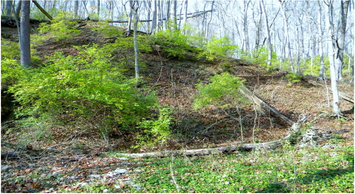
Figure AV.16: Toe of the Nordyke Road landslide.
