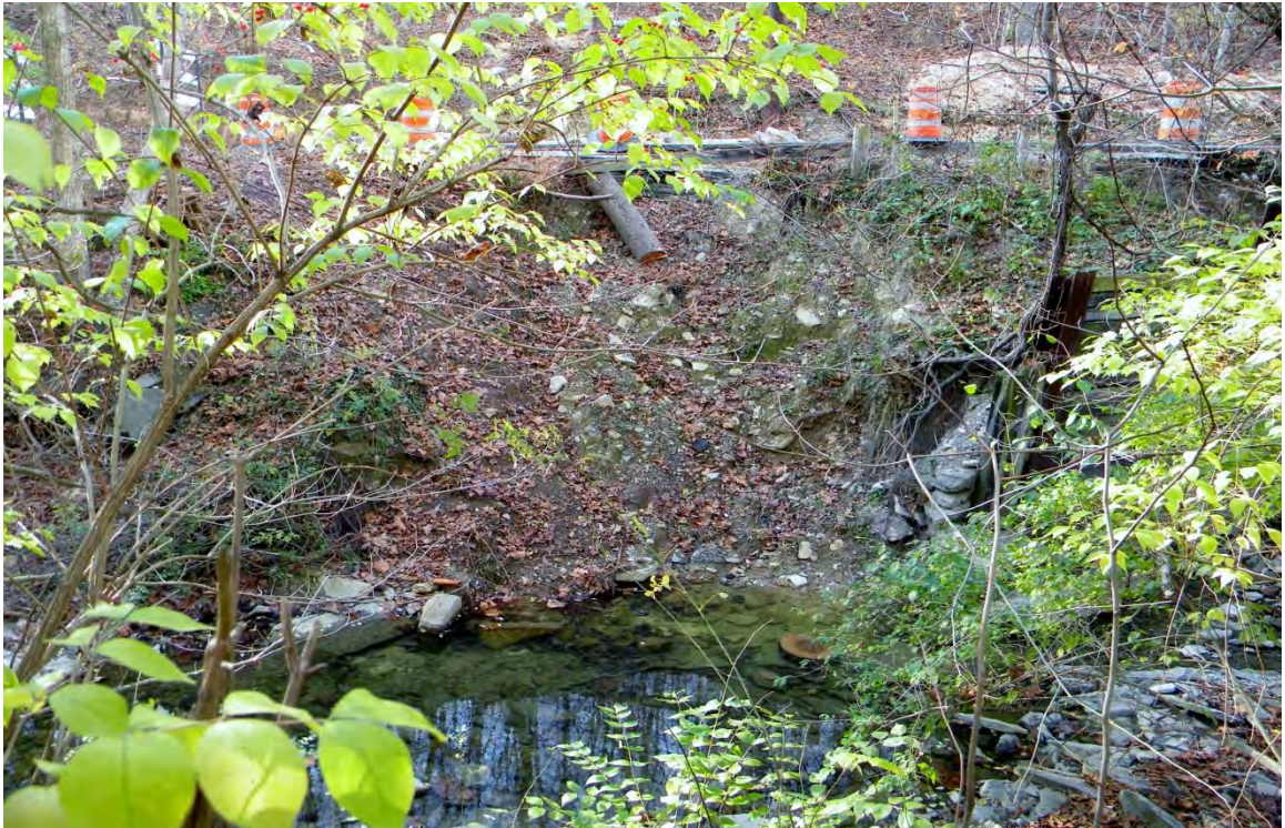
Figure AV.21: Toe at the Wagner Road landslide.
