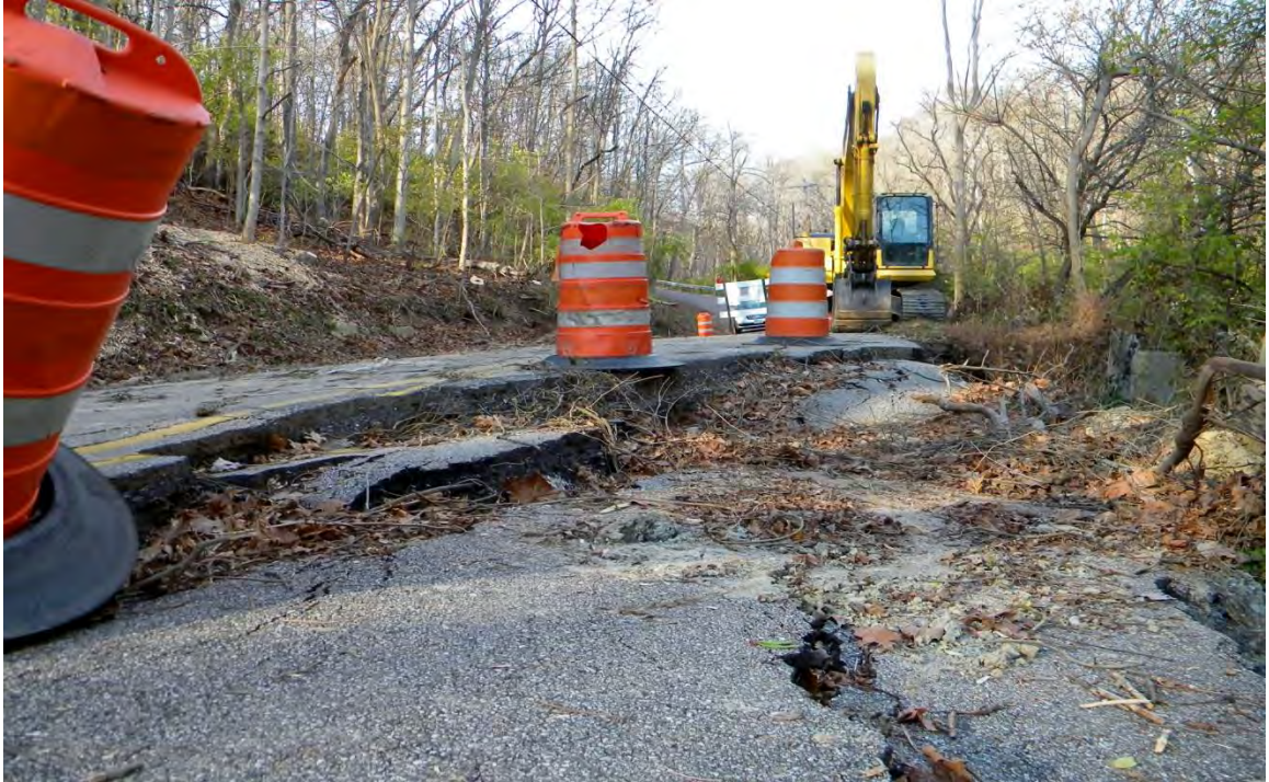
Figure AV.20: Scarp and the associated displacement at the Wagner Road landslide site.
